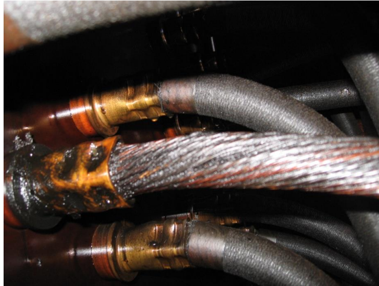
Figure 10 - Overheating of Connection #7
